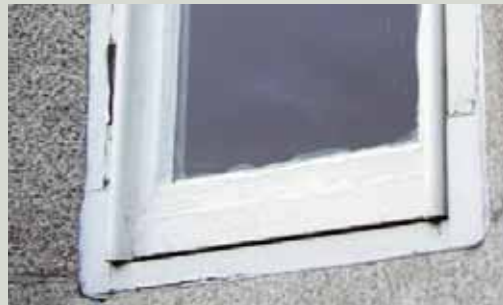
The new ends on these recently repaired stiles were not cut at an angle and the paintwork is starting to flake. Both factors will make the new joints prone to moisture ingress, which could start to damage the joint and soften the timber
