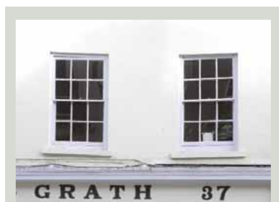
These sashes were overhauled recently, without compromising their character. It might be necessary in such cases to add timber to the stiles or rails of the sashes to line them up with the frame
