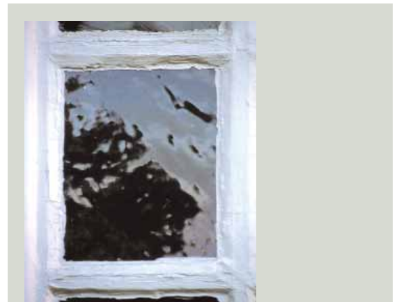
Early cylinder glass has an extremely hammered looking surface and is quite speckled with bubbles or seeds, like the pane in this early eighteenth-century window
