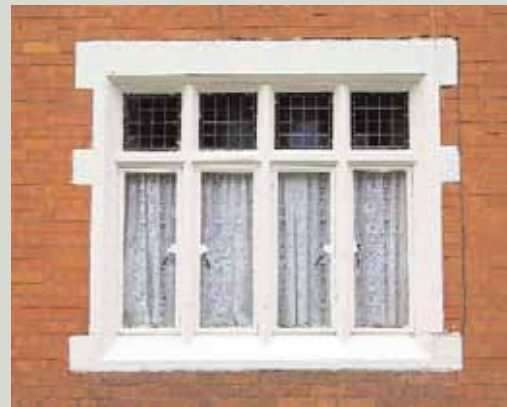
The original catches and stays survive on these metal casements. They should be retained and cared for whenever the window is undergoing maintenance, as they are an integral part of the original window
