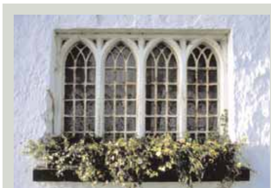
Most cast iron or steel windows contain timber sub-frames, or transoms as in this window. Sometimes the framing materials are not obvious until paint comes away and the material starts to deteriorate. It is vital to identify the framing materials when repairs are being planned
