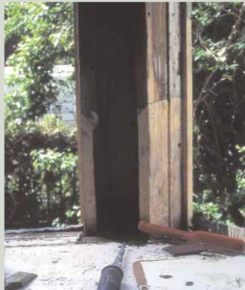
Previous repairs to the ends of this mullion were uncovered during a refurbishment project. The repairs remained in good condition and did not need attention
