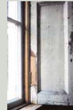
A cabinetmaker carried out some repairs to this shutter. The illustration shows new timber pieced in at the lower hinge, where decay had taken place, prior to repainting the timberwork
