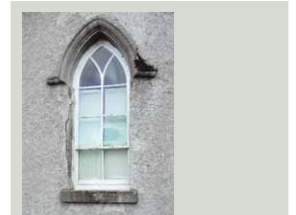
The timber in this window appears to be in reasonable condition, although repainting is required. However, the cause of the defects seen in the render beside the window and moss build-up at the hoodmould above the arch should be investigated in case they affect the window, for example by trapping moisture which could damage the timber. Any project involving this window should take especial care of the historic glass panes
