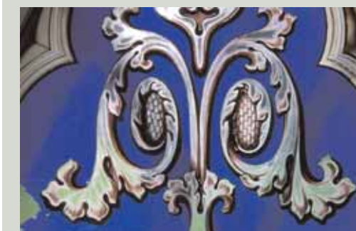
There is a diagonal crack running through this hand-painted floral panel. Even a seemingly simple matter such as gluing a crack like this is a job for a stained glass conservator, as the wrong approach could irreversibly damage the artwork
