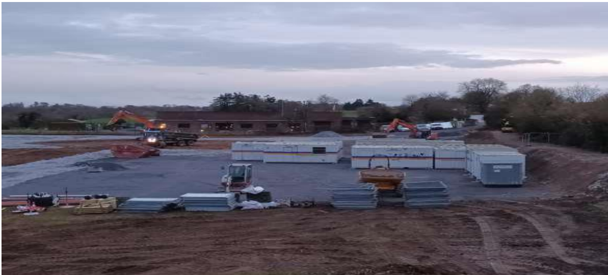
Compound setup including Safety, health and welfare facilities, offices, material storage and car parking
