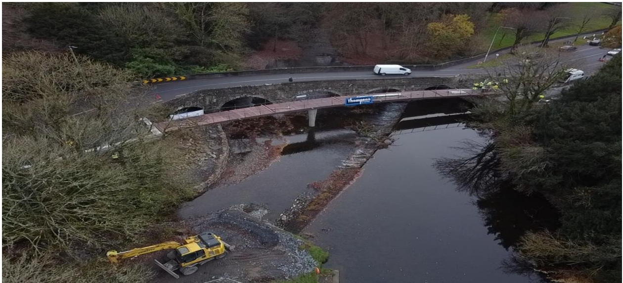
Overview with the new Castlecomer Footbridge in position (just after the bridge lift)
